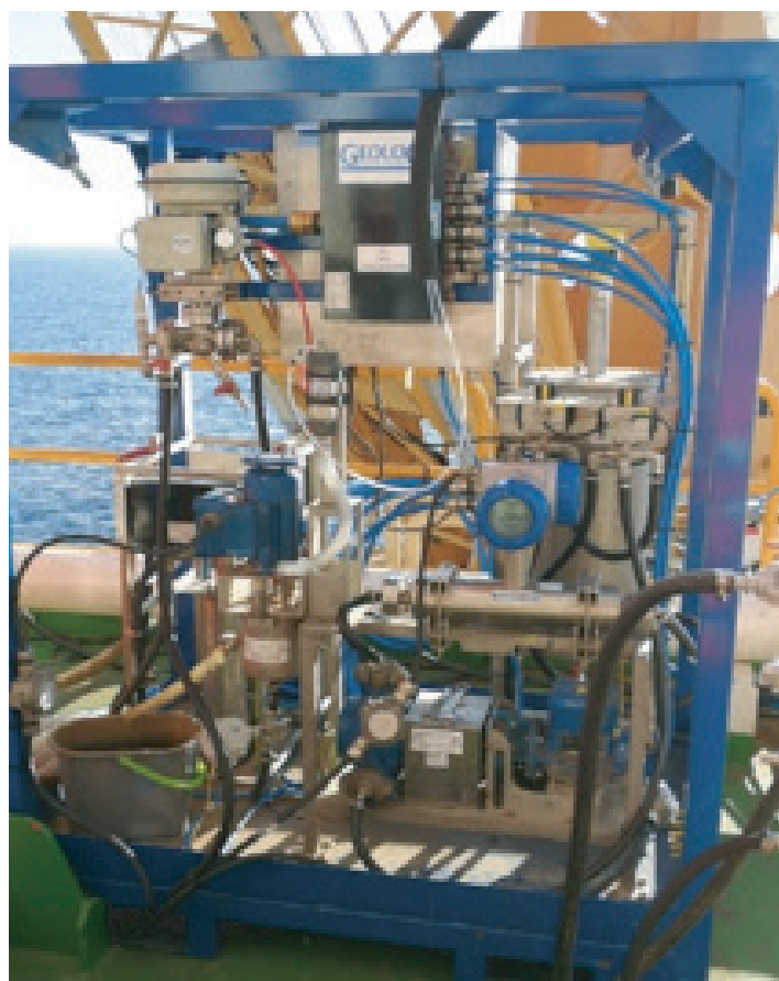
Fig.2: Pressure control, regulator and gas extractor
